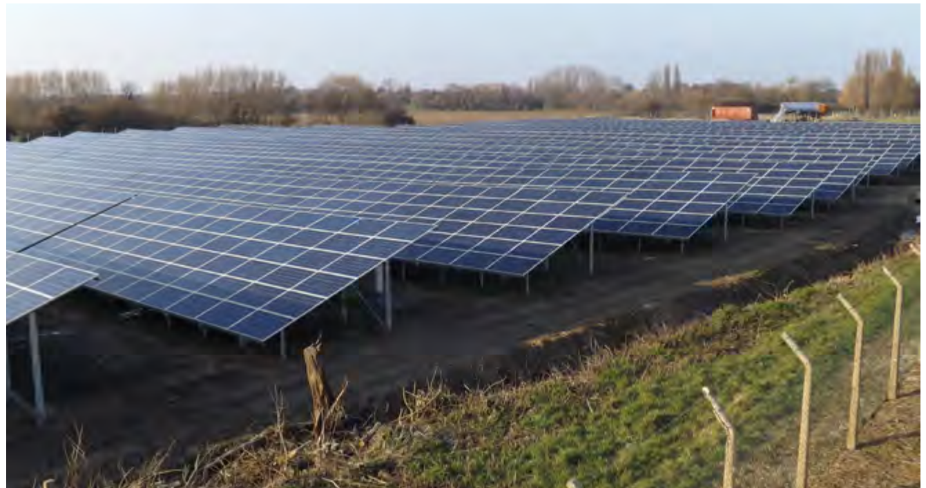
The new solar farm located at London Southend Airport which was built by Stobart Developments.
